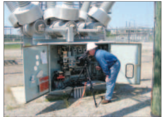
The GasFindIR LW can be used for compressor cabinet inspections and examination of other switchgear in utility situations.
