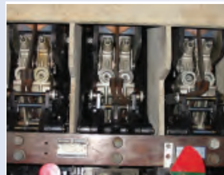
Generator Tie-In Breaker 480V
